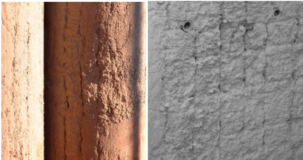
Figure E.4: Shadowing in a pile (left); mattressing in a panel (right)
