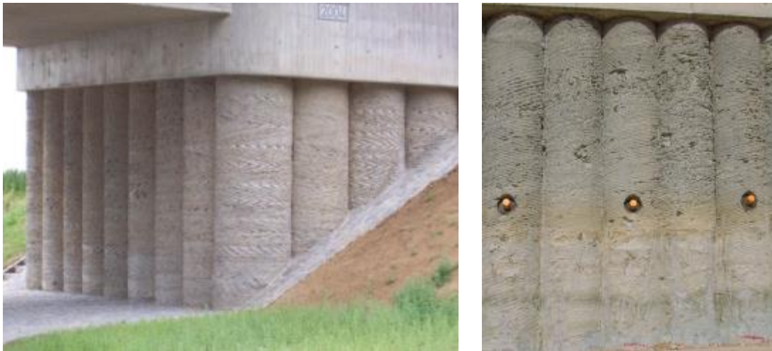
Figure E.1: Examples for piles with grooves, not affecting the minimum cover for durability
