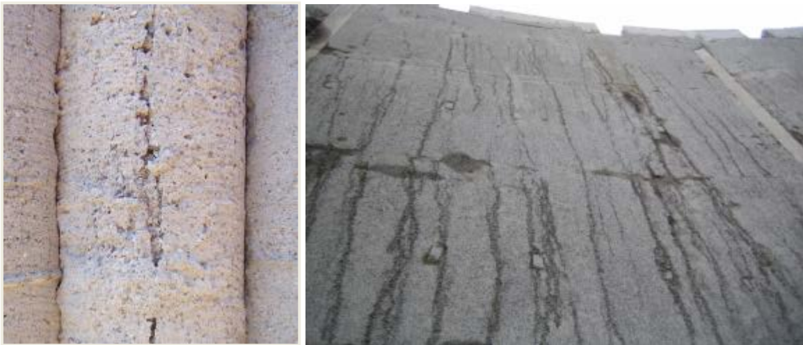
Figure E.3: Severe examples of channels running up the surface of a pile and a diaphragm wall
