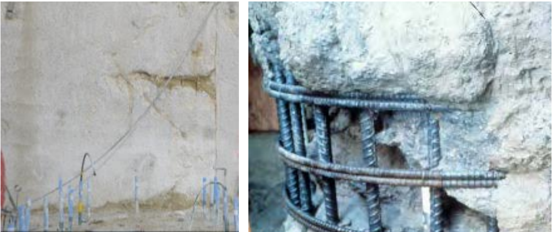
Figure E.2: Severe examples of inclusions of a diaphragm wall and a pile [pile photo taken from Figure 9.14b, FHWA GEC10]
