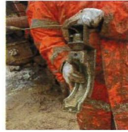
Failed clamp which attached the concrete hose to the changeover valve.
