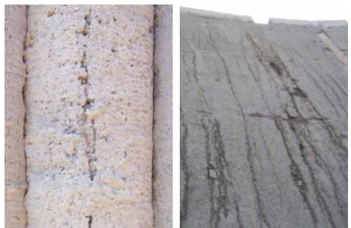
FIGURE D.4 EXAMPLES OF CHANNELS RUNNING UP THE SURFACE OF A PILE AND A DIAPHRAGM WALL
