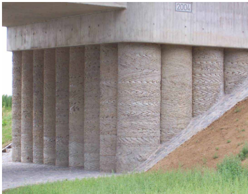
FIGURE D.1 EXAMPLES FOR PILES WITH GROOVES, NOT AFFECTING THE MINIMUM COVER FOR DURABILITY
